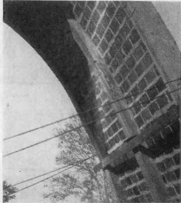
Fig. 13. Failure of middle rib. Concrete spalled from the reinforcement at the point where the bars overlapped.
